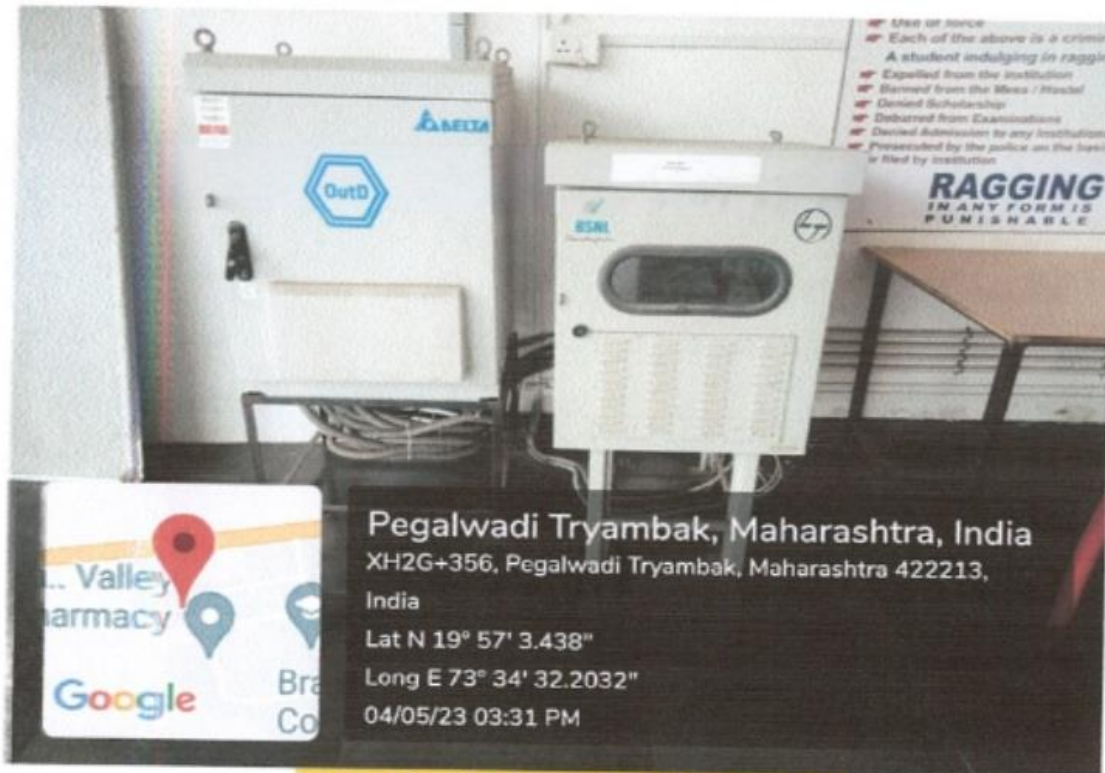
Internet Special Connection RACKS and D.P.
